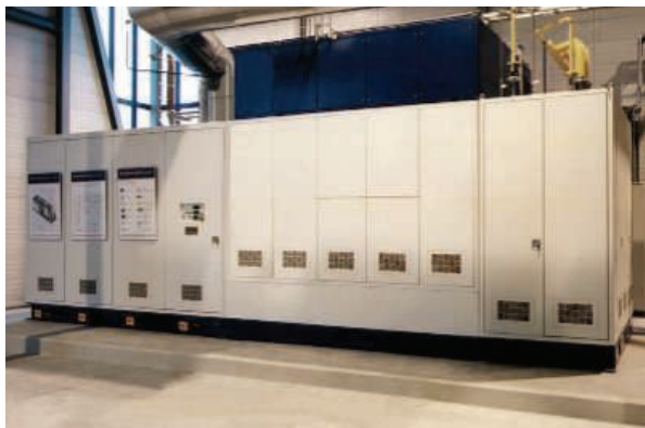
Pure and simple. Solid-oxide fuel cells, such as the ones in this 100-kilowatt heating plant in the Netherlands, require sulfur-free hydrogen.
